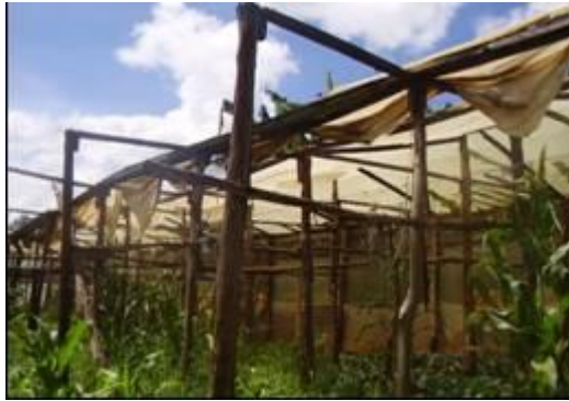
Fig. 1.a: Wrong material for construction
